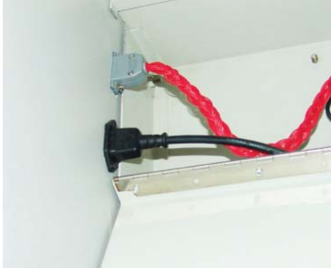
inside control box
